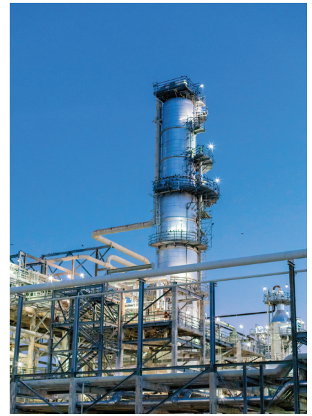
Fractionation tower in major USA refinery.
